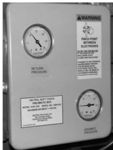
padlockable NEMA-12 regulator box
